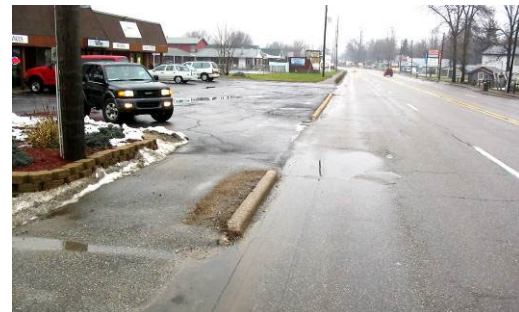
Examples of poor access management. From top: driveway spacing, parking up to pavement, poor driveway definition.
