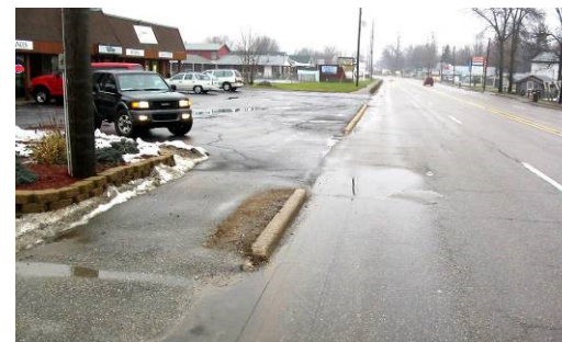
poor driveway definition
