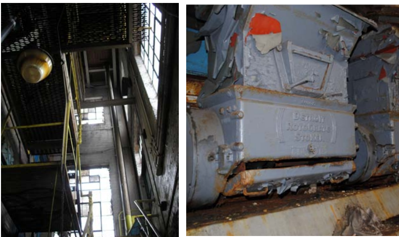
Photo 22 & 23: North-west corner and view of hazardous equipment
