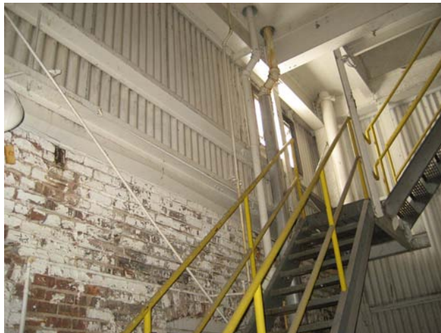
Photo 39: Interior shows steel walls built on top of the remains of building 4
