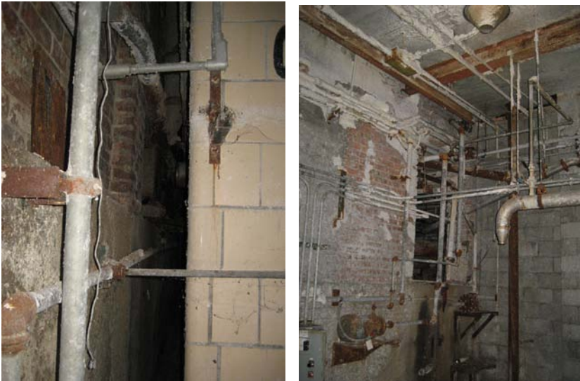
Photo 48 & 49: Views of the exterior wall of building 3 and seam of building connection
