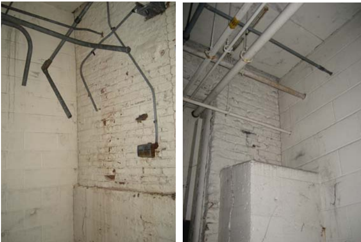
Photo 43 & 44: Views of seams where buildings are attached
