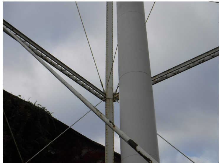
8) The sway rods are in good condition. The coating is in poor condition.
