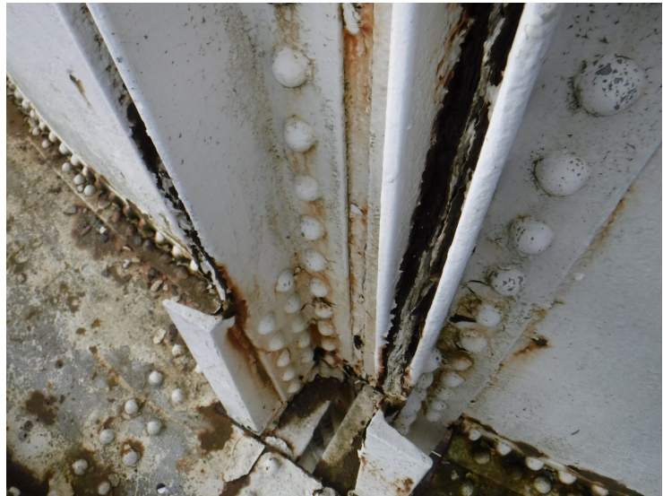
14) The leg to bowl connection is in poor condition. There is active corrosion in the crevices.
