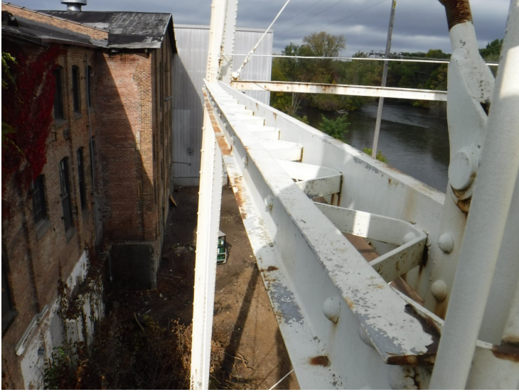
10) Typical strut is in good condition. The coating is in poor condition.
