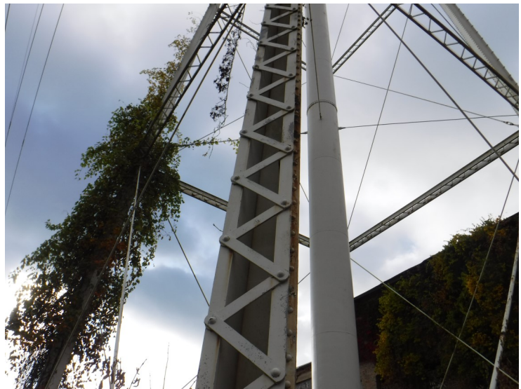
5) Typical lattice leg is in good condition. The coating is in poor condition.
