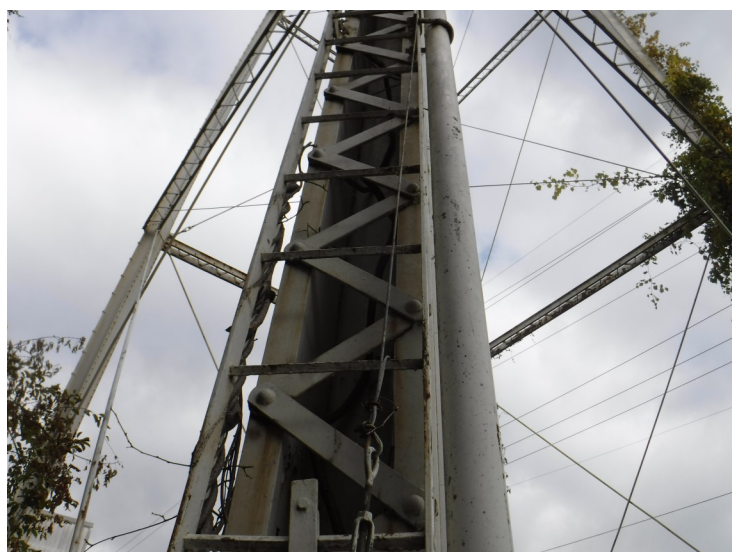
9) The leg ladder is in good condition. The ladder is equipped with a cable-type fall prevention device that is undersized.
