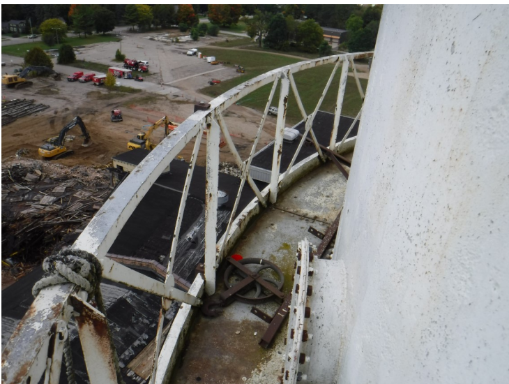
12) The balcony is in fair condition. The coating is in poor condition.
