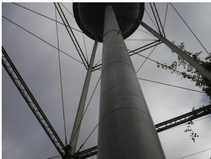
6) The riser is in good condition. The coating is in poor condition.
