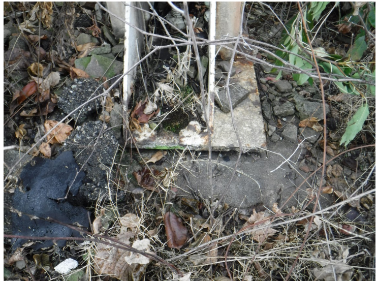
2) Missing grout underneath a leg.
