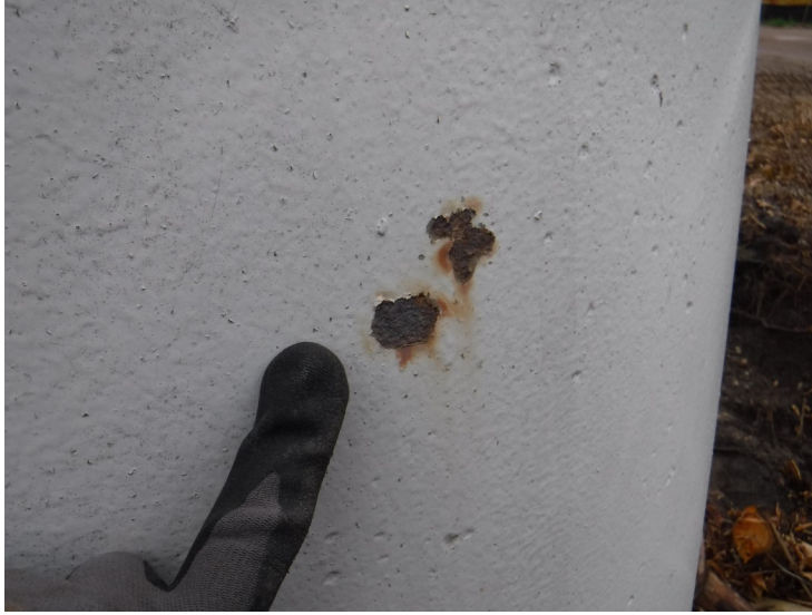
7) Coating failures on the riser.
