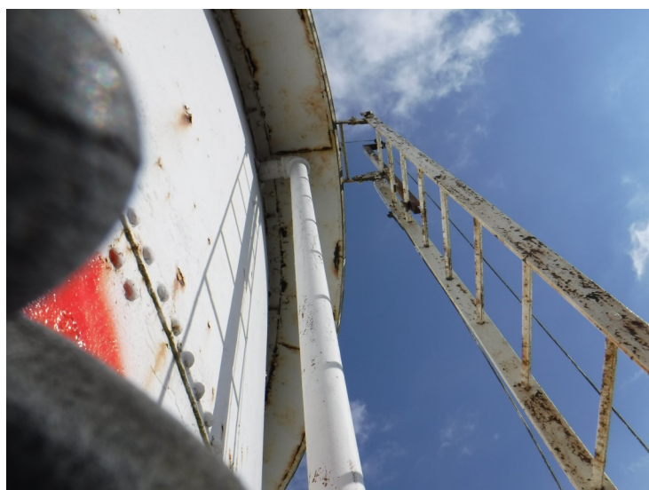
18) The rotating sidewall ladder is in fair condition. The ladder is equipped with a cable-type fall prevention device that is undersized.
