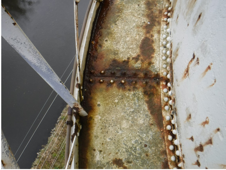
13) There is evidence of water ponding on the balcony. There is active corrosion occurring on the floor plates.
