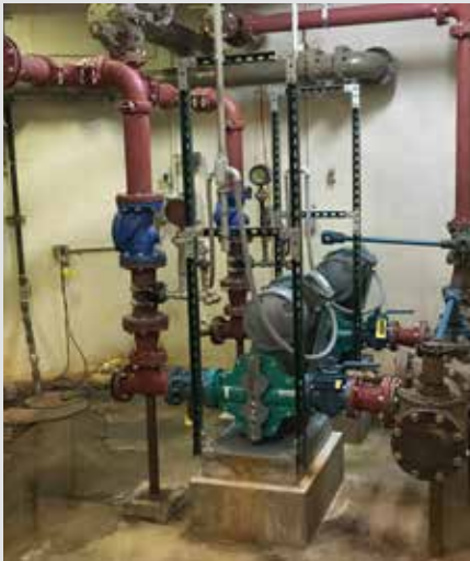
The City of Otsego WWTP installation of NETZSCH TORNADO® T2 Rotary Lobe Pumps.
