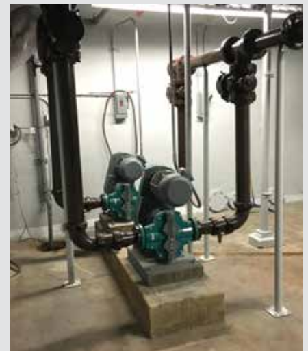
The NETZSCH TORNADO® T2 Rotary Lobe Pumps in the Plainwell Water Renewal facility requires only a small footprint while providing easy access for maintenance.
