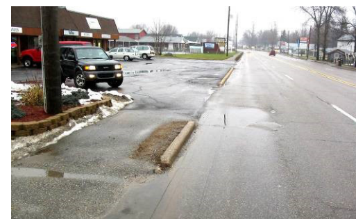
poor driveway definition
