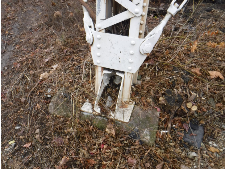
1) Typical leg is in good condition overall. The foundation concrete is in good condition.
