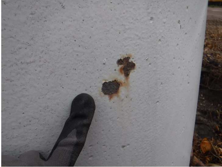
7) Coating failures on the riser.
