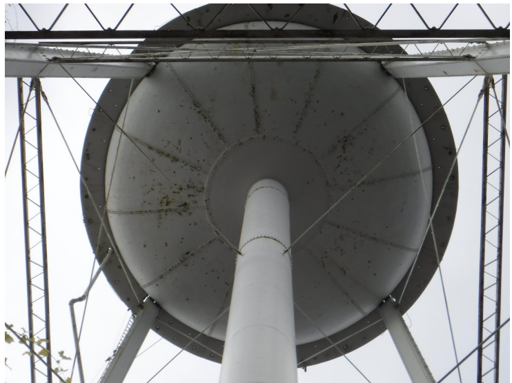
11) The bowl is in good condition. The coating is in poor condition.
