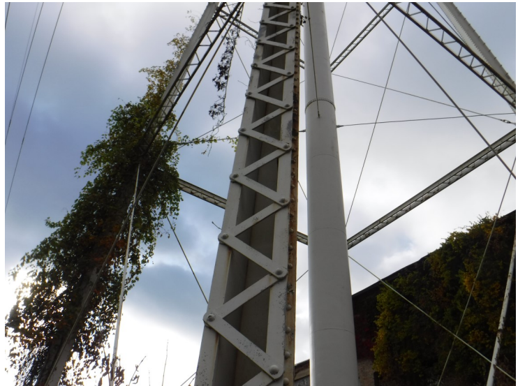
5) Typical lattice leg is in good condition. The coating is in poor condition.
