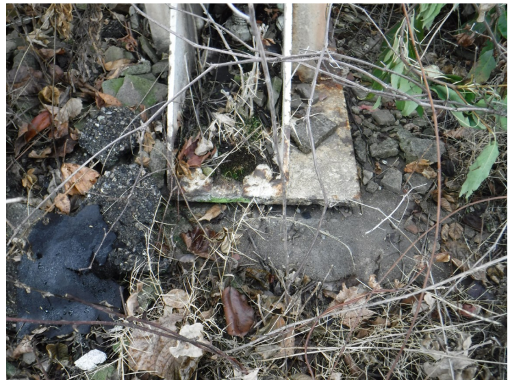
2) Missing grout underneath a leg.
