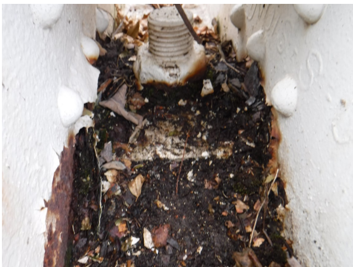
3) Active corrosion of leg anchor bolt and nut.
